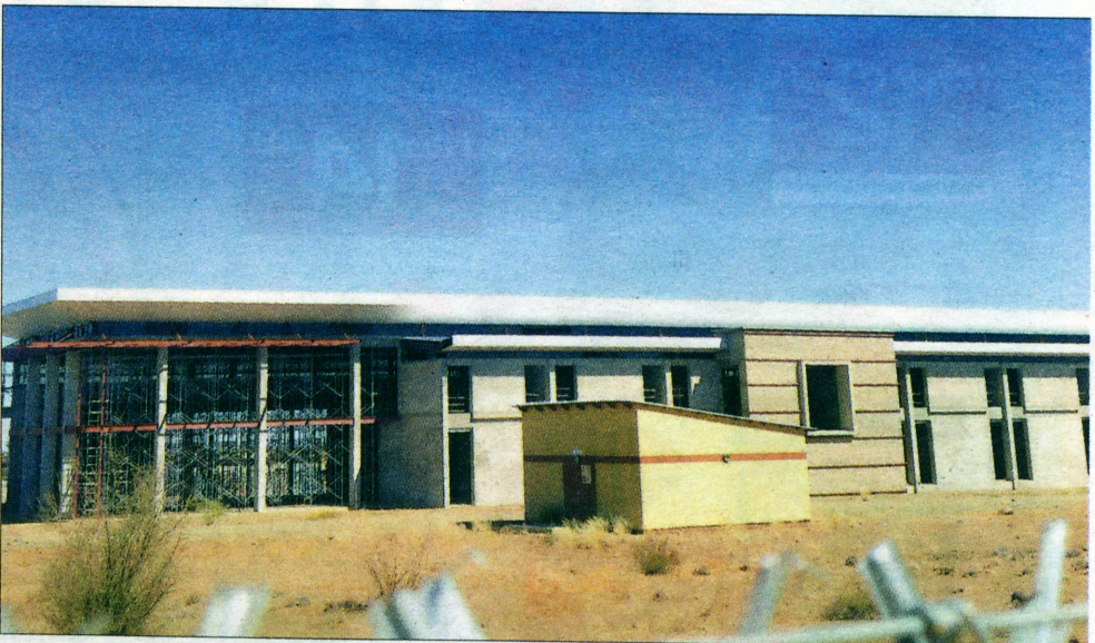
INCOMPLETE ... The incomplete Unam southern campus building at Keetmanshoop.
